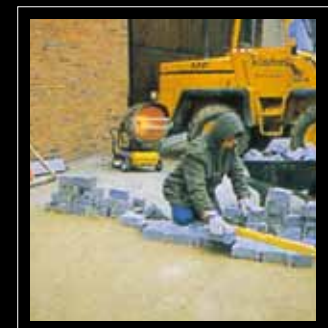
Warms up machines and personnel Winter construction: heats up materials, machines, and working sites
